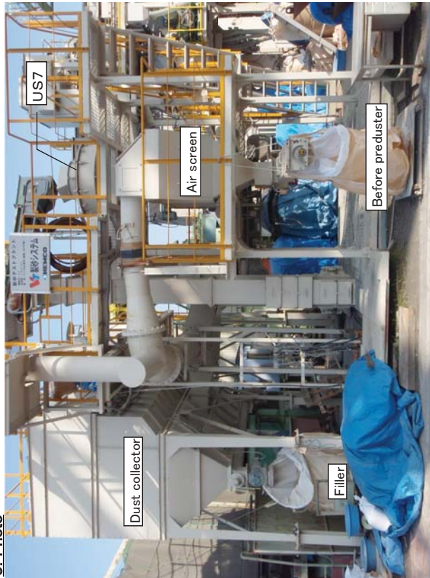
a) V7 test plant
