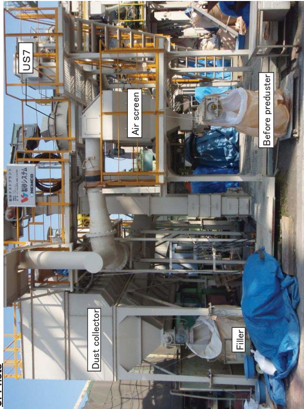
a) V7 test plant
